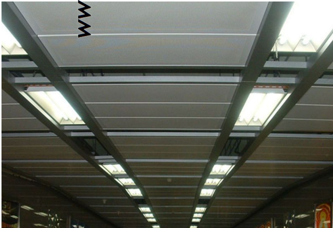
Perforated Panels as ceiling.(acoustic ceiling)
