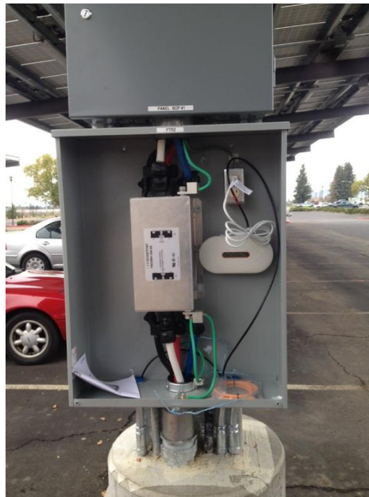
Figure 6 Aftermarket Filter for a Solar Parking Lot
