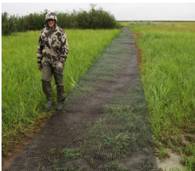
Long time Refuge user Julie Burt walks the trail line along the freshly placed Geo-block® underlayment.
