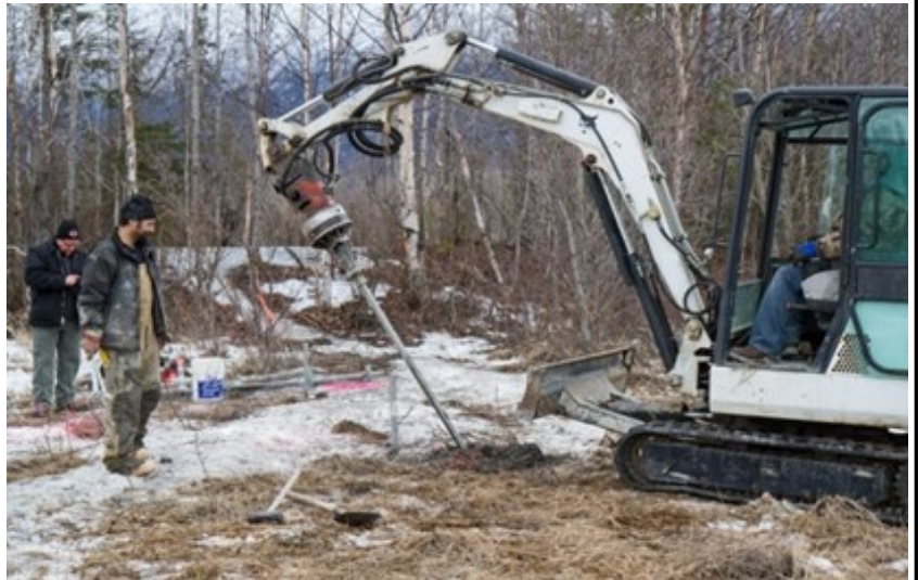
Alaska Foundation Technology staff torque in the 45° "batter" pile to link with the vertical pier. Special Inspector Mark Dean stands in the background.
