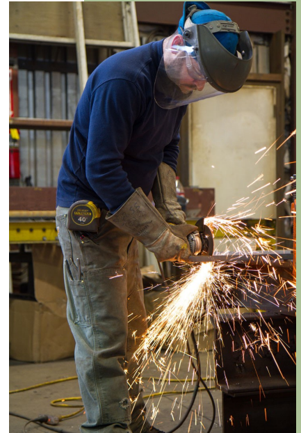
Sampson's Johnathan Bass creates guard rail verticals from bar stock prior to welding the Tower's safety grab rail features.
