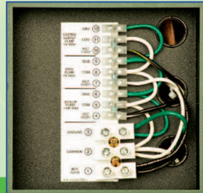
High Voltage Wiring Center (rear of boiler)
